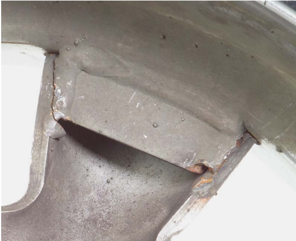
Closer view still, of weld failures.
