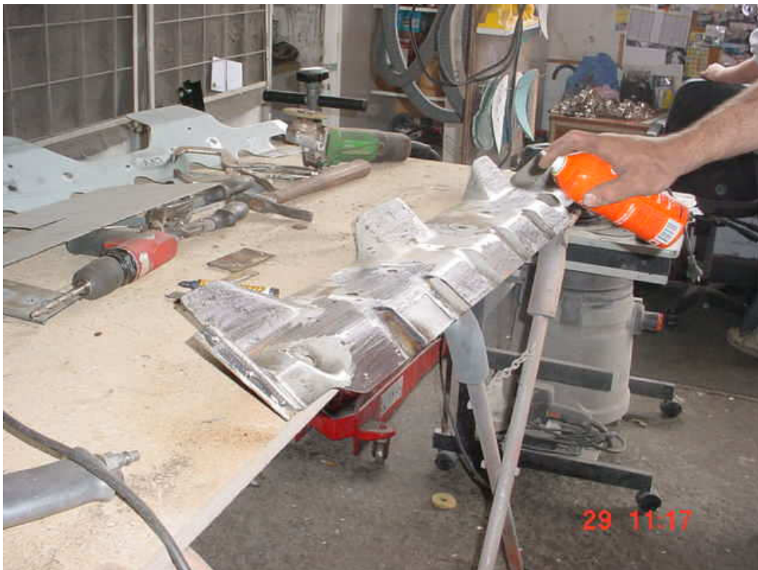
Apply corrosion converter/epoxy primer to all bare metal on the reinforcer plate.
