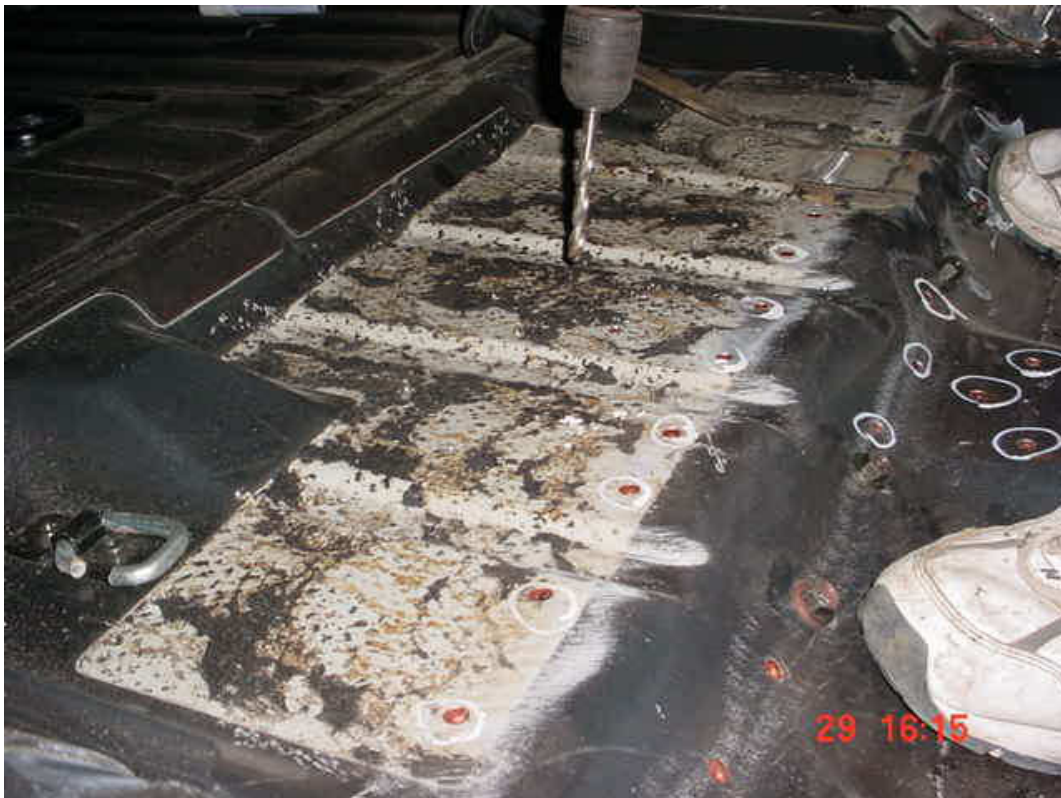
From inside the vehicle, open out the sixteen 2 mm holes just drilled. Drill 8 mm (5/16") through the floor (one layer), these are now ready for plug-welding. Fit some PK screws and panel washers to pull the plate assembly firmly against the floor if necessary. Plug-weld all holes. AJ
