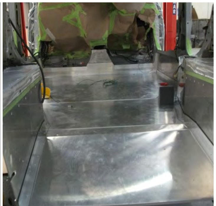
Above: The new aluminium sandwich panel floor, looking toward the front of the vehicle, creating a smooth unobstructed path for a wheelchair occupant.
